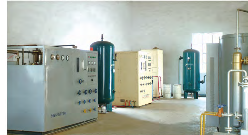
氨分解炉和制氮机 AMMONIA DECOMPOSITION MACHINE AND NITROGEN GENERATOR
